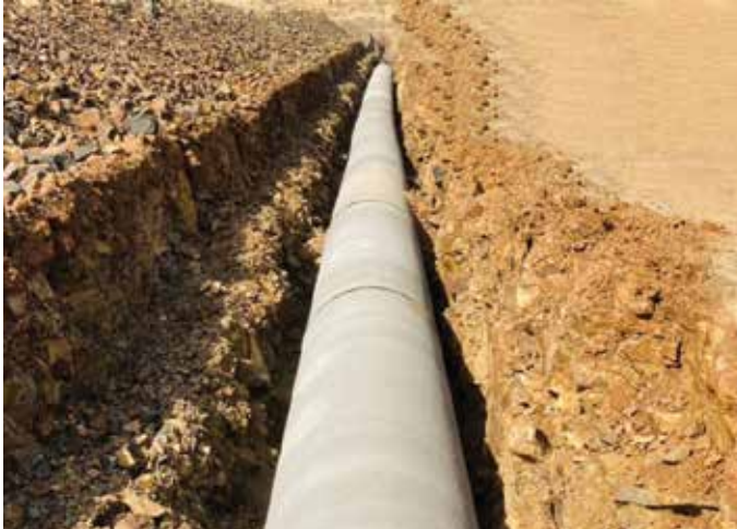
1000 mm dia PCCP pipeline laying work at Man Canal PDN of Urmodi Irrigation Project in Maharashtra
