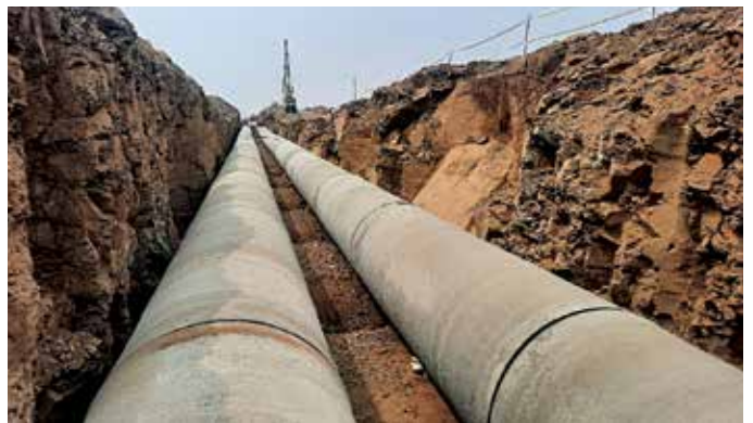
Supply of 1700 mm dia PCCP pipes for Jath Lift Irrigation Scheme, Sangli, in Maharashtra
