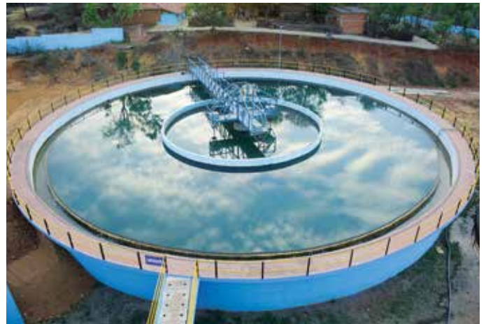
20.60 MLD Water Treatment for Kandaila Multi Village Rural Water Supply Scheme in Rewa District in Madhya Pradesh.
