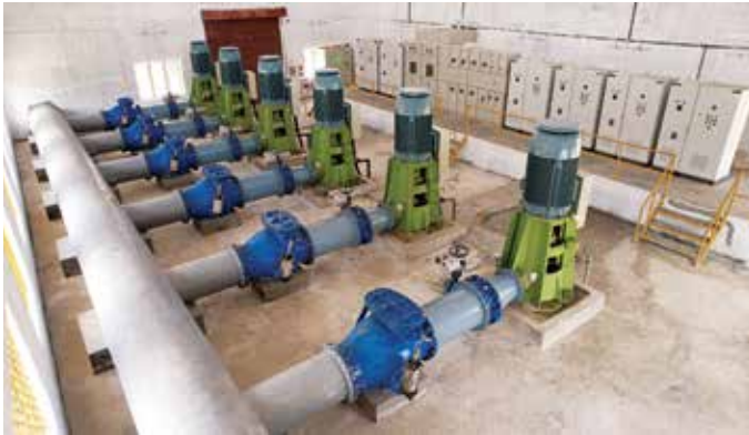
23555 lpm x 16.30 Mtr head VTPS - 6 Nos at Head works at Dedicated Water Supply Scheme package-I for Madurai Corporation in Tamil Nadu
