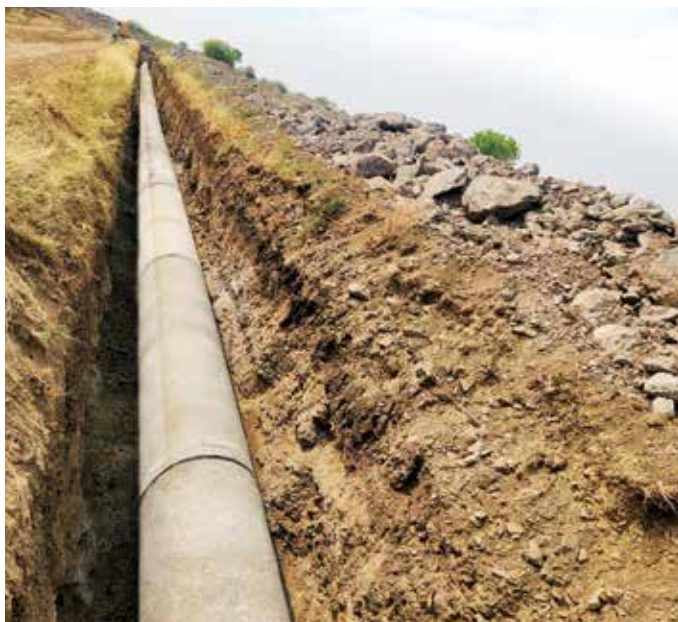
1000 mm dia PCCP pipeline laying work of Dahigaon LIS PDN for Solapur Irrigation Division in Maharashtra.
