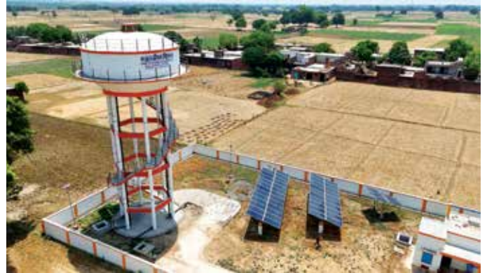
Tube Well cum Pump House, 20 KW Solar Power Plant and 200 KL Over Head Tank at Ikorapur, Auraiya District for Kanpur Water Supply Scheme (SWSM) in Uttar Pradesh
