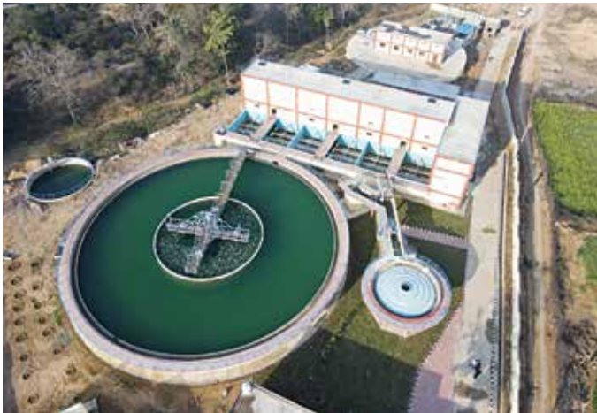
25 MLD Water Treatment Plant for Kuraicha Water Supply Scheme in Uttar Pradesh.
